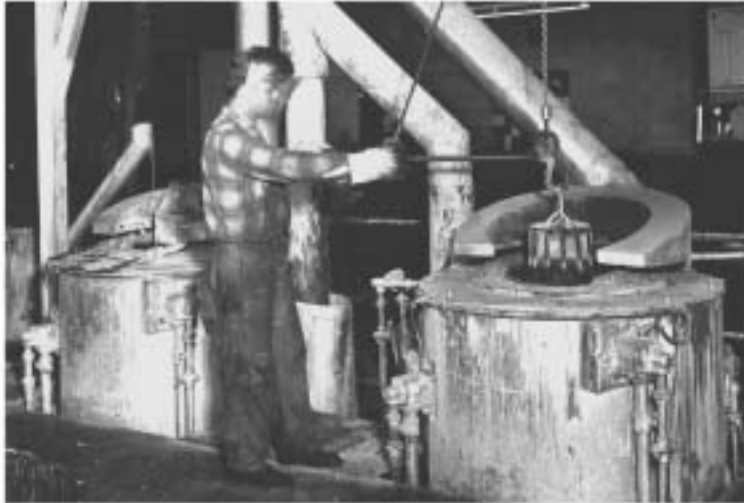
423-3-A Burners firing salt posts dramatically demonstrate they are designed for severe service conditions.
